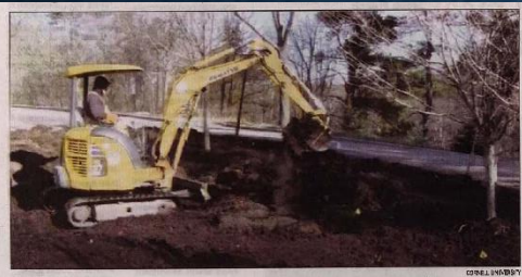
A backhoe breaks up compacted soil as part of a research project undertaken by the Cornell School of Horticulture.
